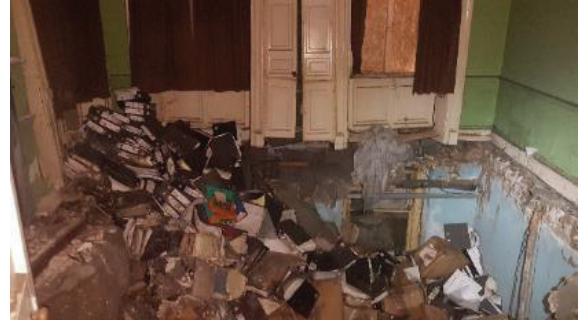
Figure 10.6: Partially collapsed floor
