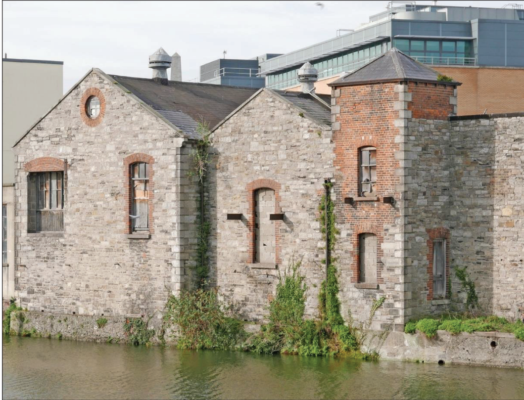
Figure 12.15: Square Tower on the Riverfront – seen here to the right of the image
